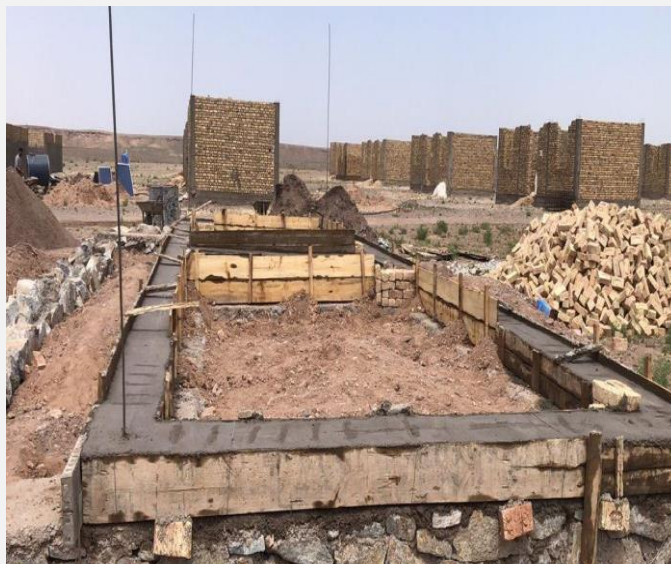
Supported by IFRC, ARCS constructs demo shelters in Gulran district, Herat province. (Photo: Meer Abdullah Rasikh, IFRC)
