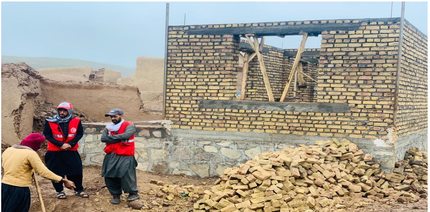
ARCS supported by IFRC, provides construction material, cash and technical assistance to households displaced by the earthquake in Gulran district of Herat province. Specifically, ARCS/IFRC is supporting the construction of 300 owner-driven houses in Herat province.
